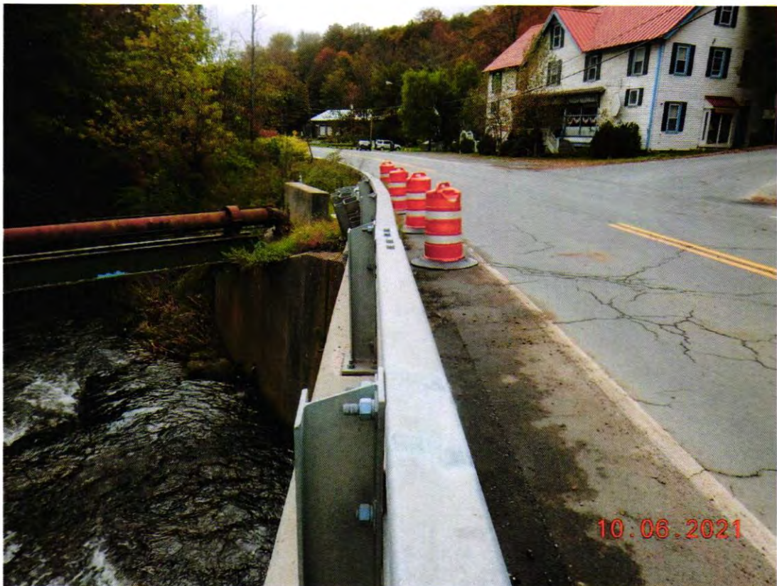
October 2021 No Movement of barrier
