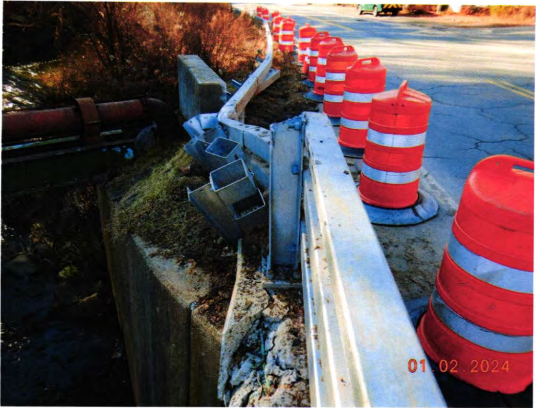
January 2024 No Movement of barrier
