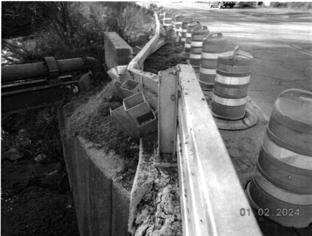
January 2024 No Movement of barrier
